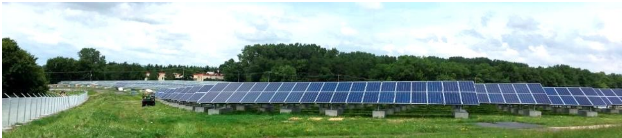
Barr played a key role in the installation of a 3,000-panel solar farm on top of a closed landfill without impact to the landfill's cover and integrity.
